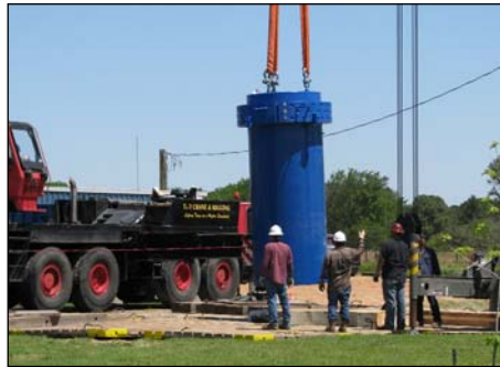
Arrival and Installation of New Pressure Vessel at SEA CON Advanced Products, LLC
