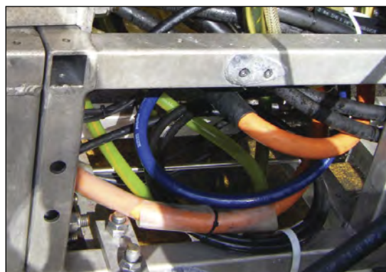
Figure 9: PBOF hose constraints on intervention skid
